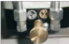
By pass valves Valves by-pass
