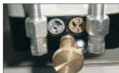
By pass valves Valves by-pass
